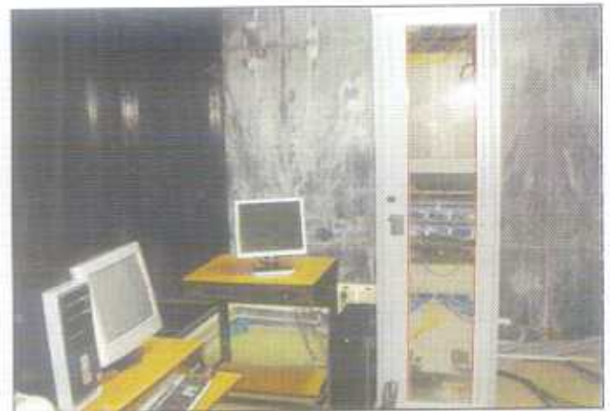
IT Infrastructure at CMC
